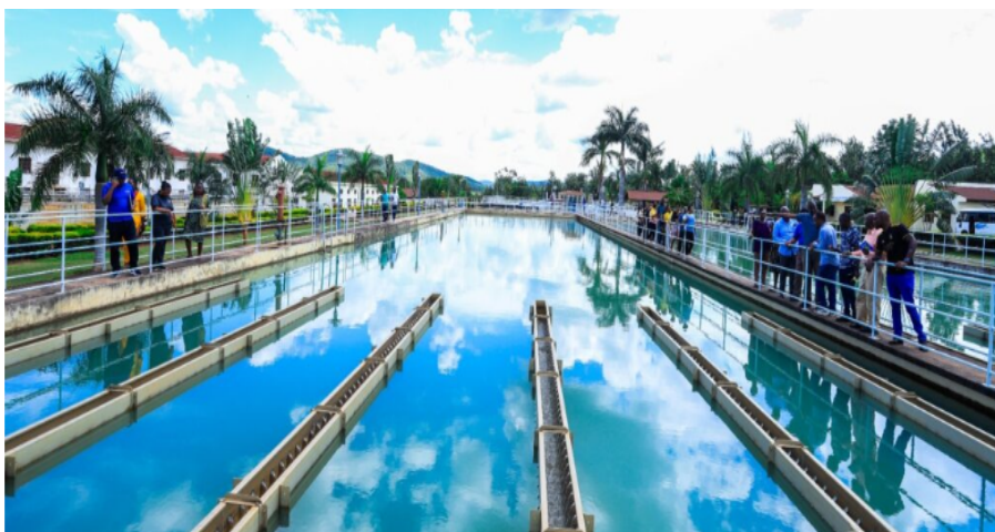
Figure 3.1: Lake Victoria water production facility, Ihelele - Mwanza
